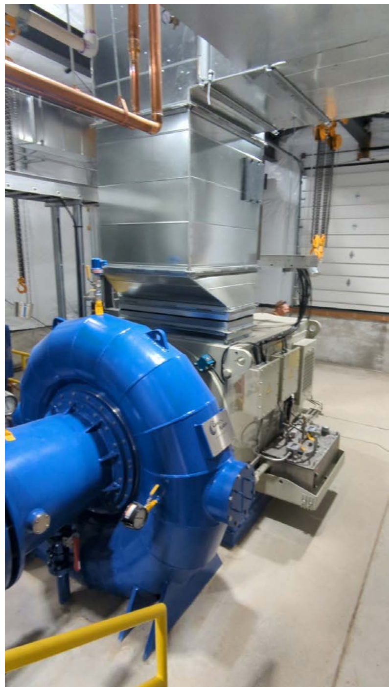
The Taylor River Hydro Project turbine and generator.
