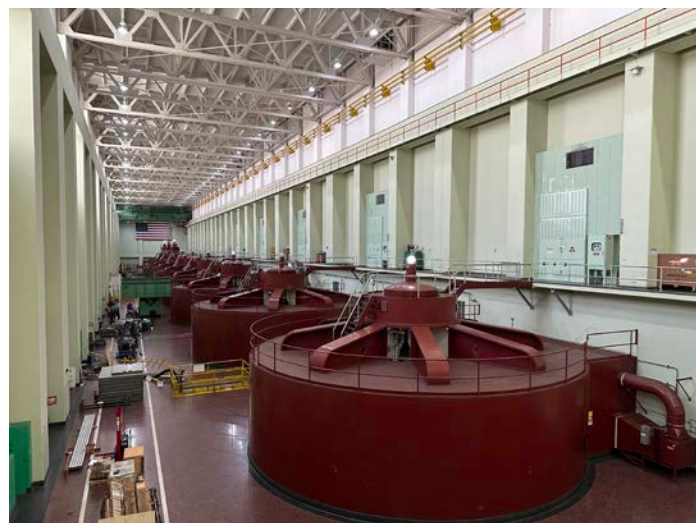
The Nathaniel "Nat" Washington Powerhouse at Reclamation's Grand Coulee Dam.
