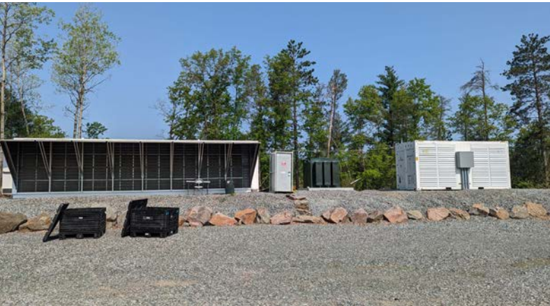
The DPO-operated bitcoin mining facility in Hatfield, Wisconsin.
