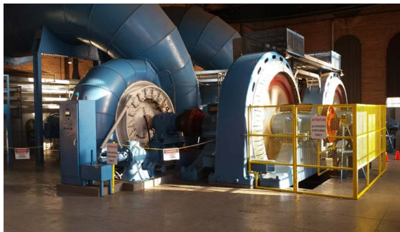
Turbines and generators inside the powerhouse at the facility in Hatfield.
