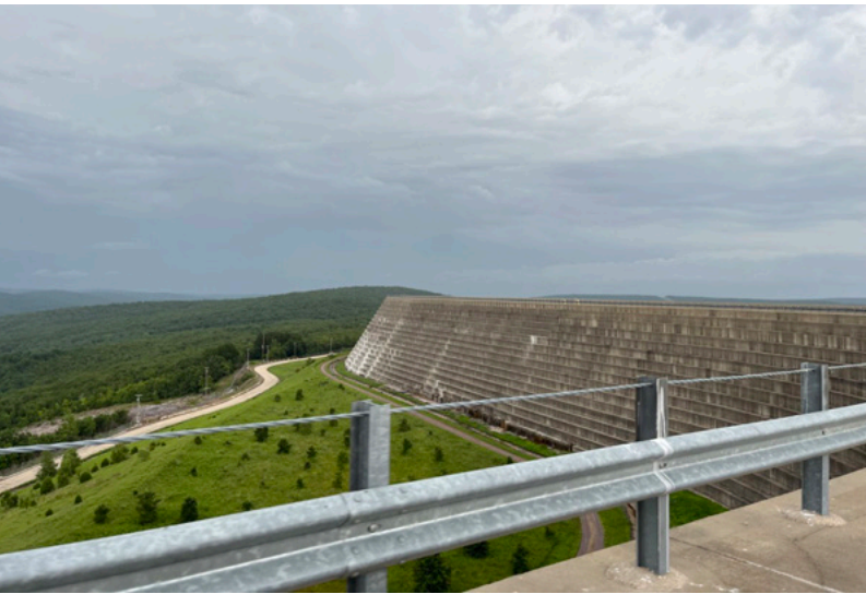
A photo taken during a daily inspection of Taum Sauk Pumped Storage Project in Missouri, conducted by GZA and the site operator in support of the external owner's dam safety program.
