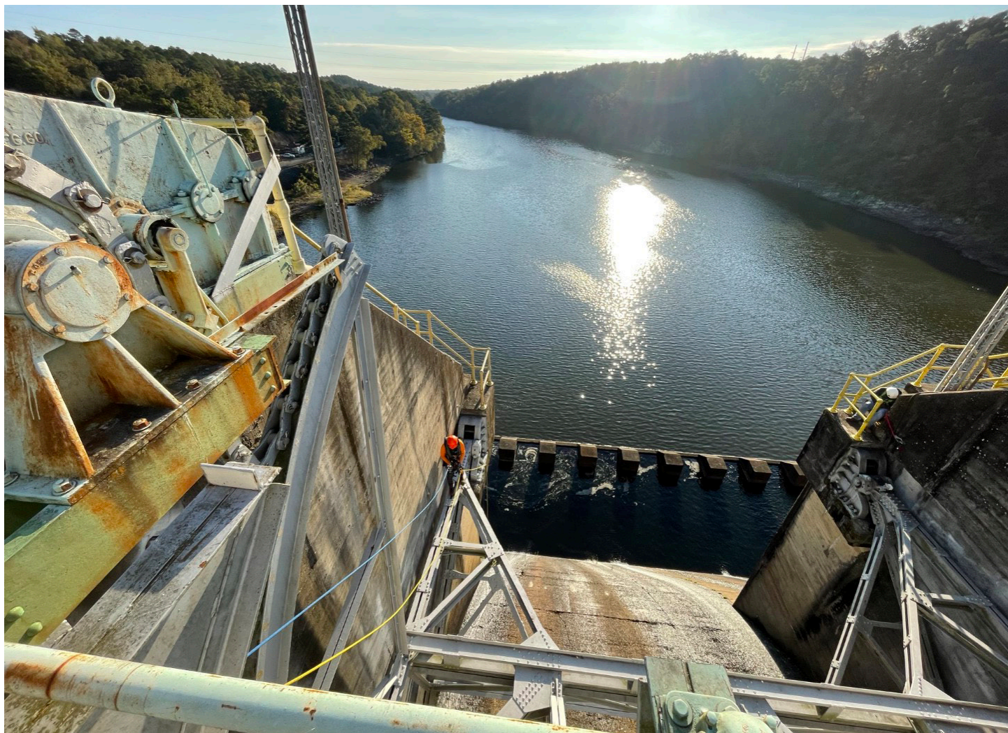
A GZA technician performs a rope-access inspection of the spillway tainter gates at the Rempel Development in Arkansas.
