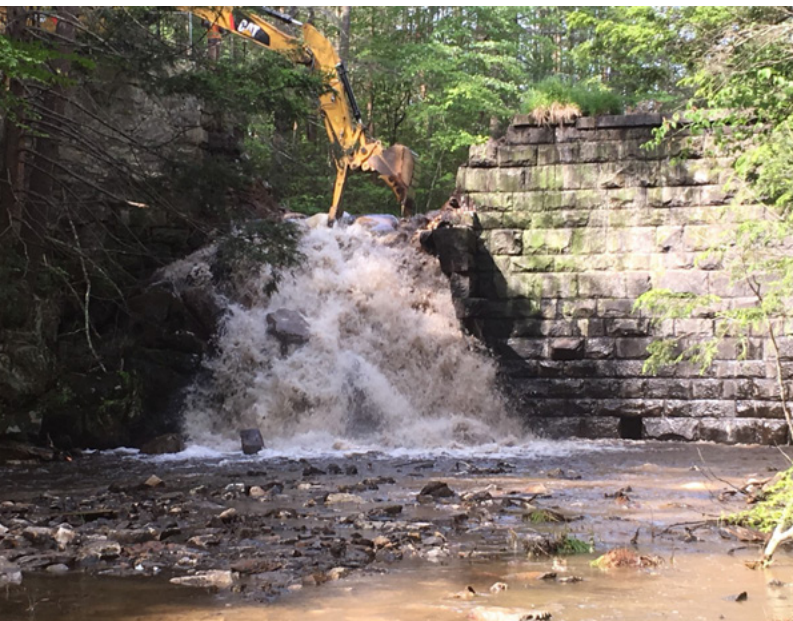
GZA performed the investigations, alternatives analyses, preliminary and final design, environmental permitting, and construction phase engineering services for the removal of the Upper Roberts Meadow Reservoir Dam in Northampton, Massachusetts.
