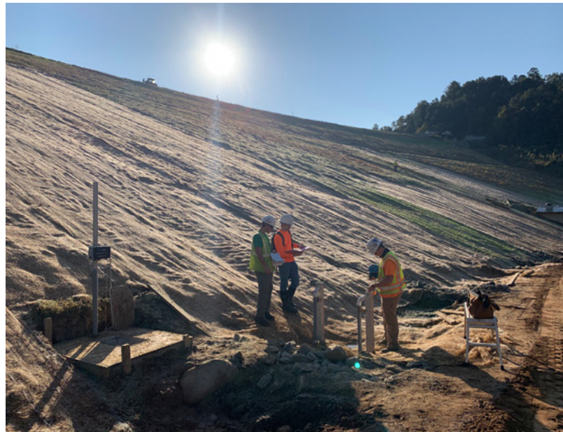
GZA field staff initializes and installs vibrating wire piezometers and an automated data acquisition system at the North Fork spillway and embankment improvements project in Black Mountain, North Carolina.
