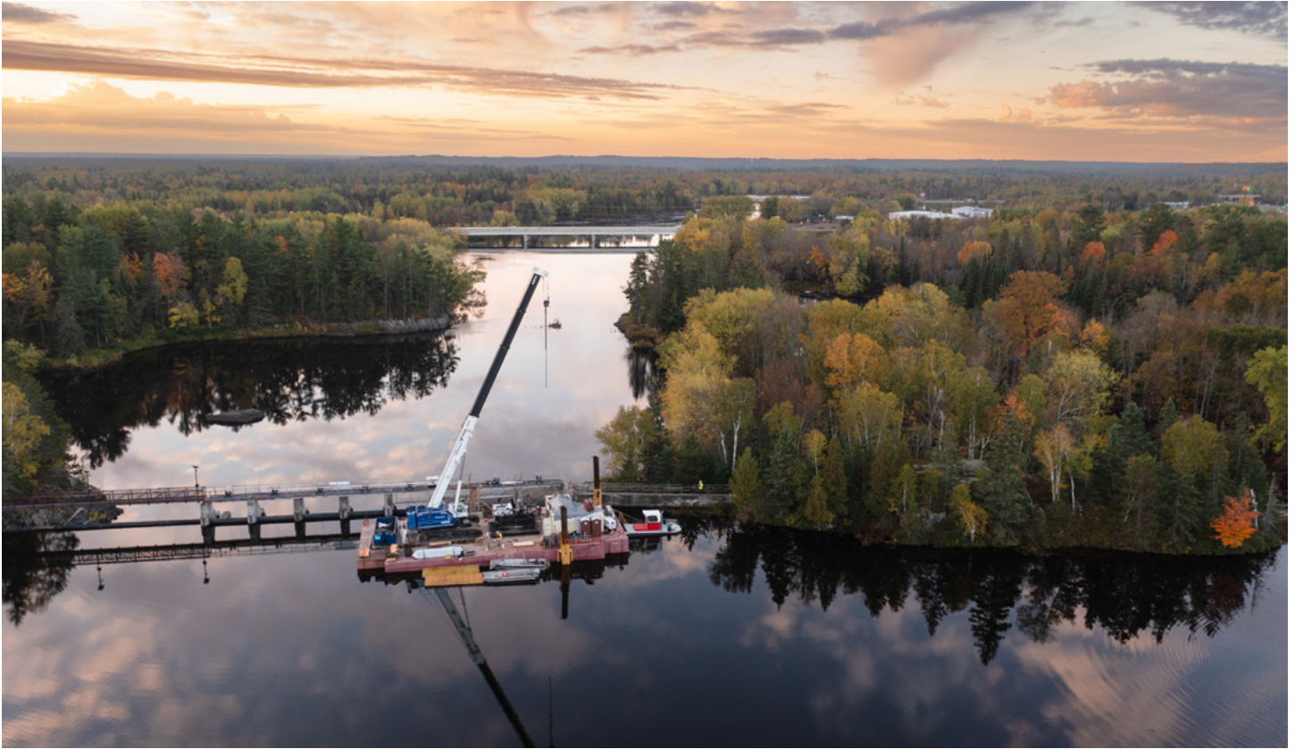
The J.F. Brennan Company works on the restoration of Scanlon Dam in Scanlon, Minnesota.
