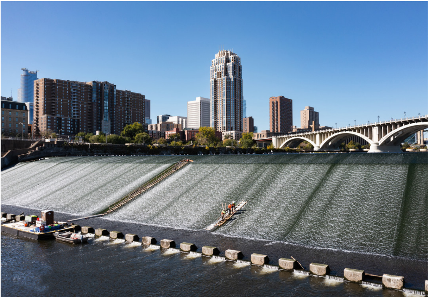
Brennan works to repair the St. Anthony Falls Spillway in Minneapolis, Minnesota.
