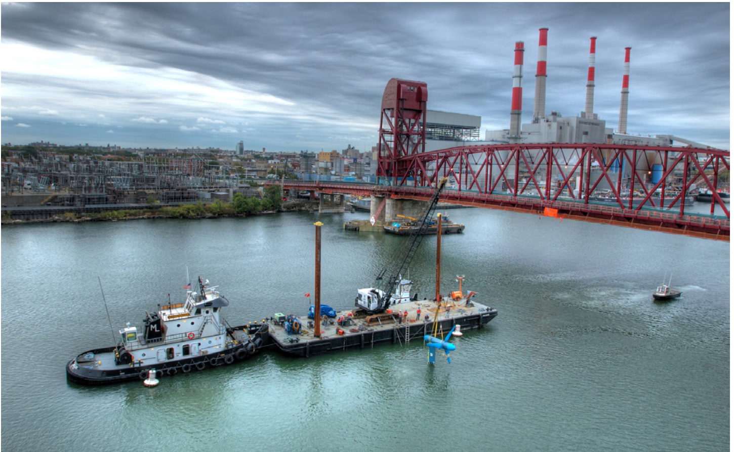
The installation of a Verdant Power tidal turbine at the Roosevelt Island tidal energy site in New York.
